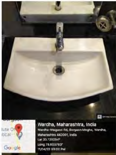
Taps to be replaced by faucets
