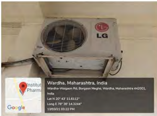
AC Condenser in shade
