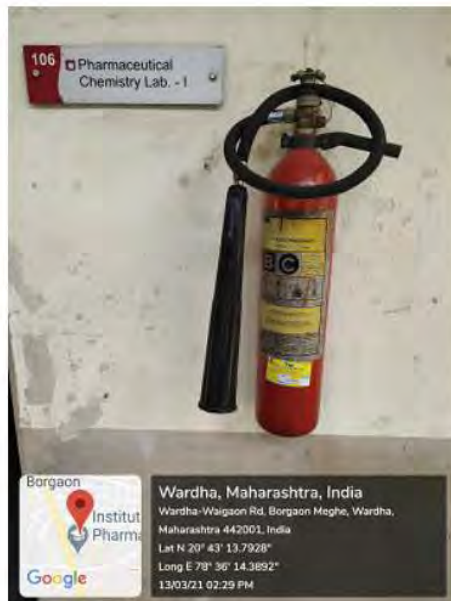
Fire Fighting System installed in college
