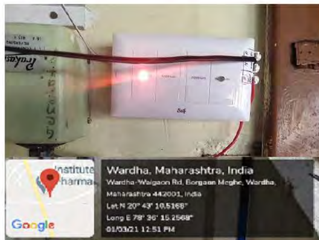
Sensor based lighting installed in college
