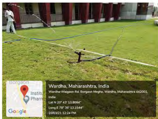
Sprinkler System installed in college for gardening
