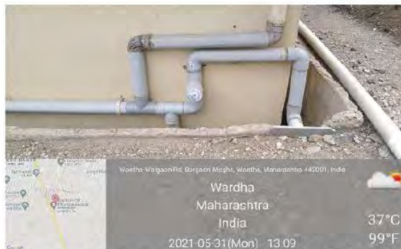
Water filtration unit connected to Water Harvesting Pit
