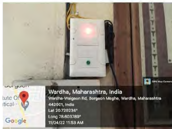
Sensor based lighting installed in college
