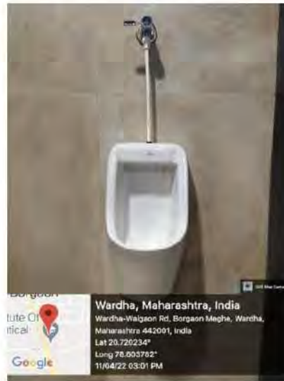
Valves to be replaced by push buttons
