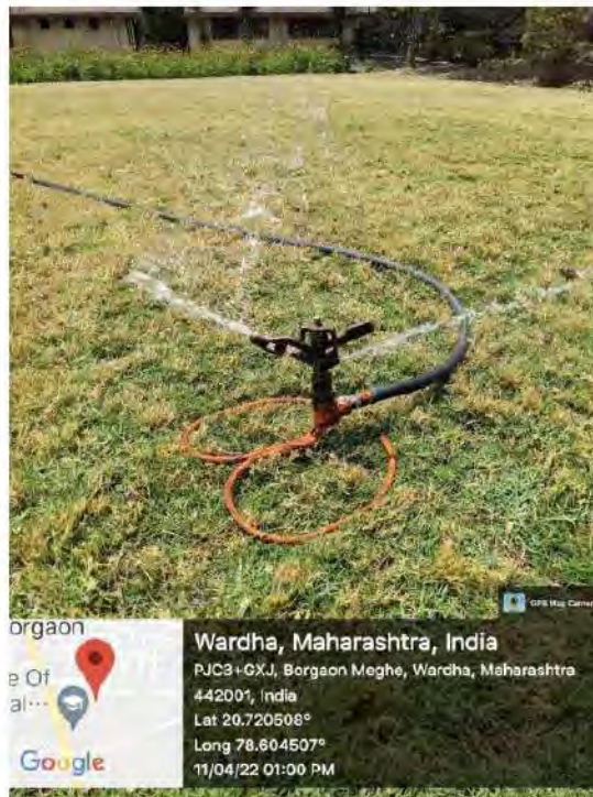
Sprinkler System installed in college for gardening
