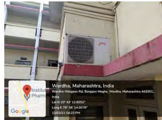
AC Condenser exposed to direct sunlight
