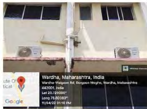
AC Condenser exposed to direct sunlight
