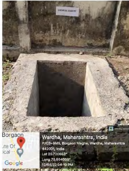
Chemical waste soak pit
