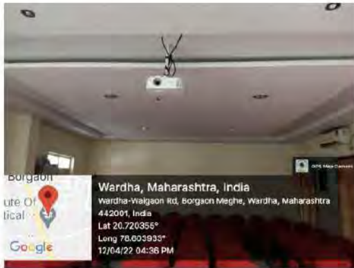
Use of false ceiling to reduce air-conditioned volume and reducing AC load
