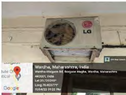
AC Condenser in shade
