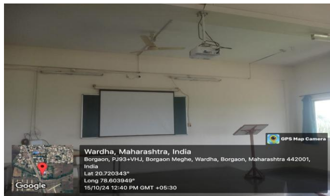
LCD ROJECTOR- BENQ INSTALLED IN ROOM NO 314
