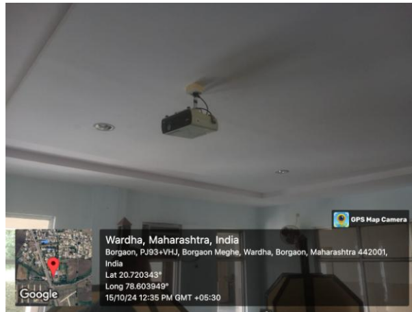
LCD PROJECTOR – EPSON INSTALLED IN ROOM NO. 215
