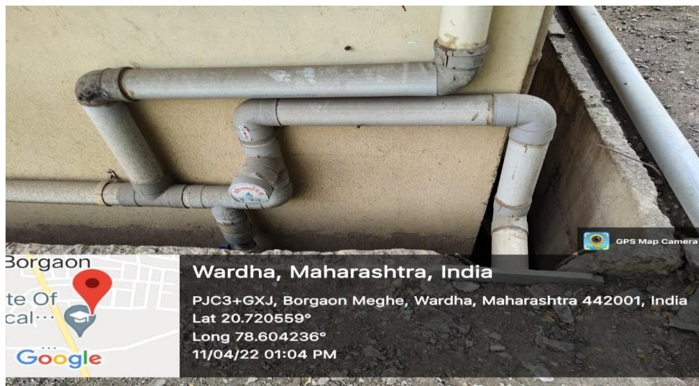
Water filtration unit connected to water harvesting pit
