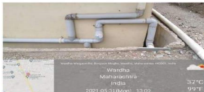
Water filtration unit connected to Water Harvesting Pit
