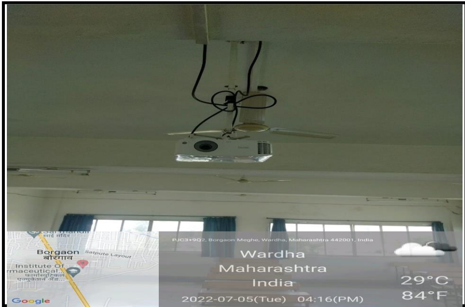
LCD ROJECTOR- BENQ INSTALLED IN ROOM NO 311
