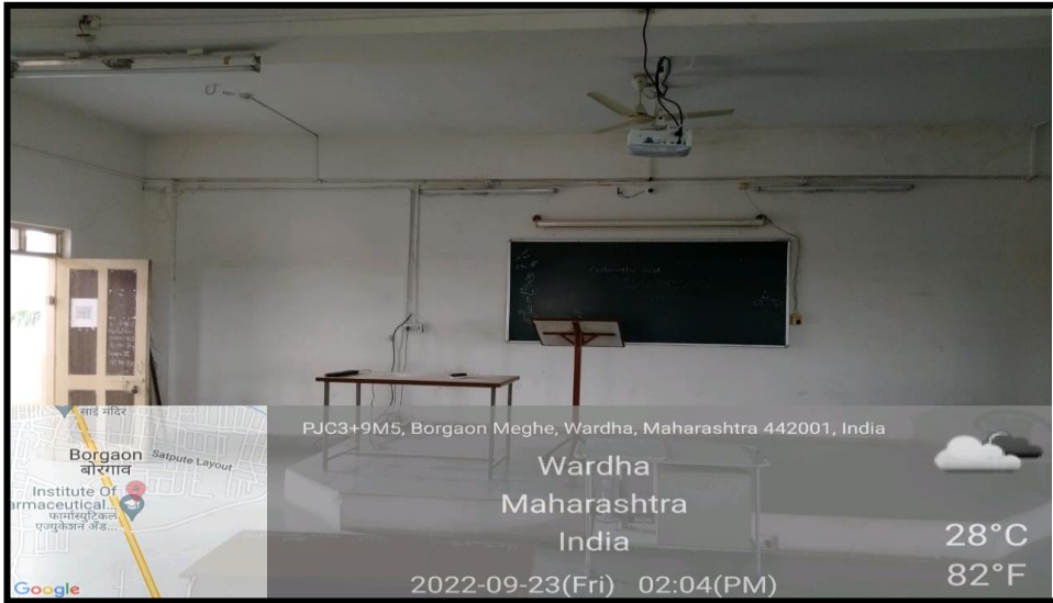
LCD ROJECTOR- BENQ INSTALLED IN ROOM NO 314
