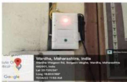
Sensor based lighting installed in college
